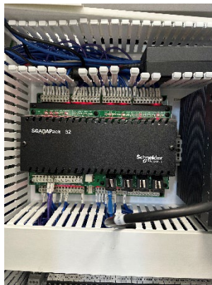
Remote Well No. 5
