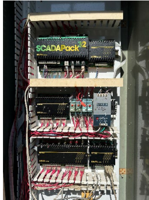
Remote Well No. 3
