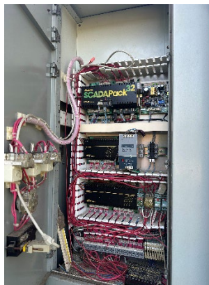
Remote Well No. 4
