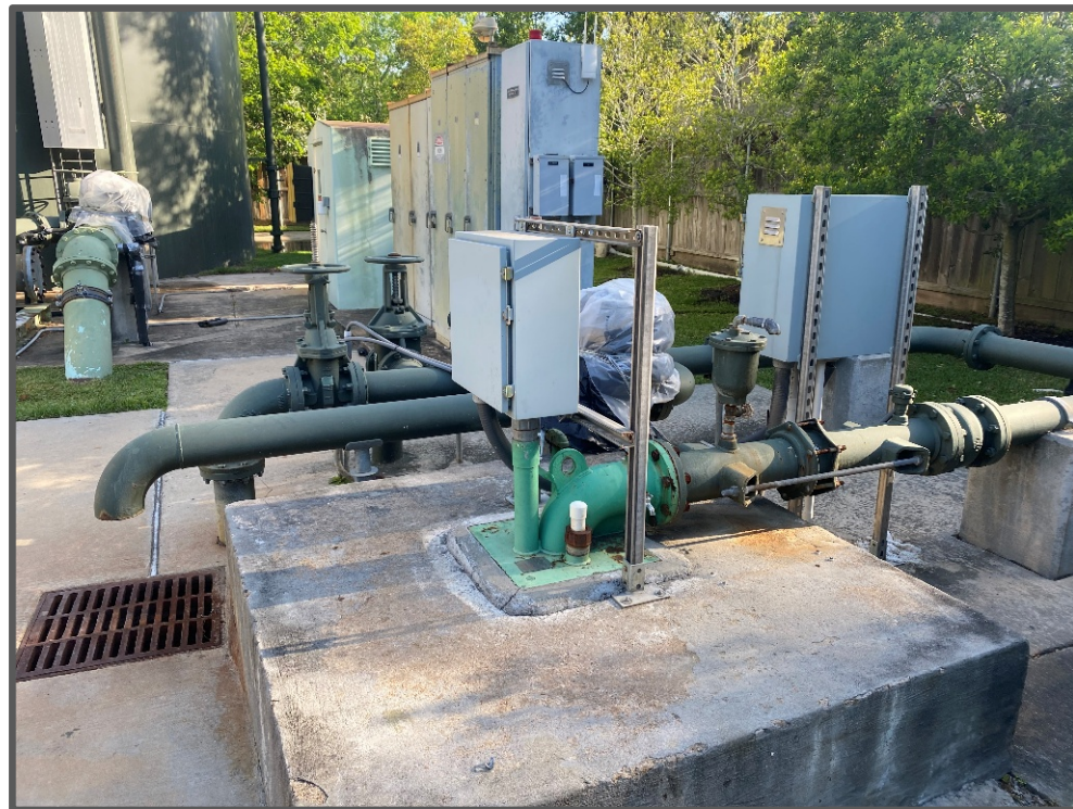
WP No. 1 On-Site Well (Water Well No. 1) and Electrical Equipment
