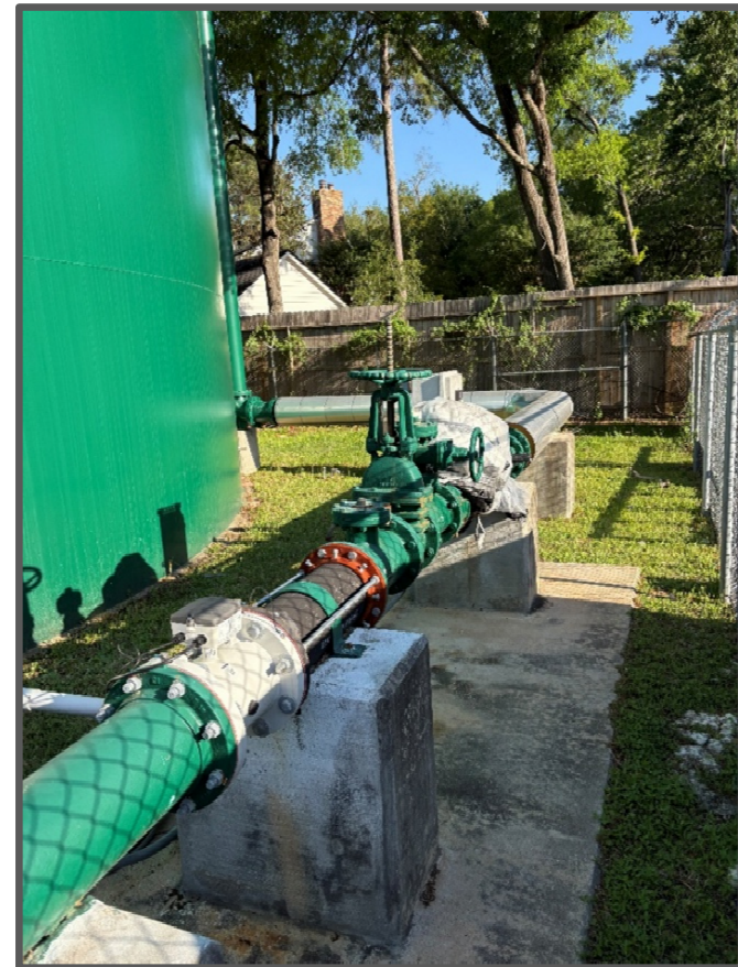
Surface Water Meter Station at WP No. 2
